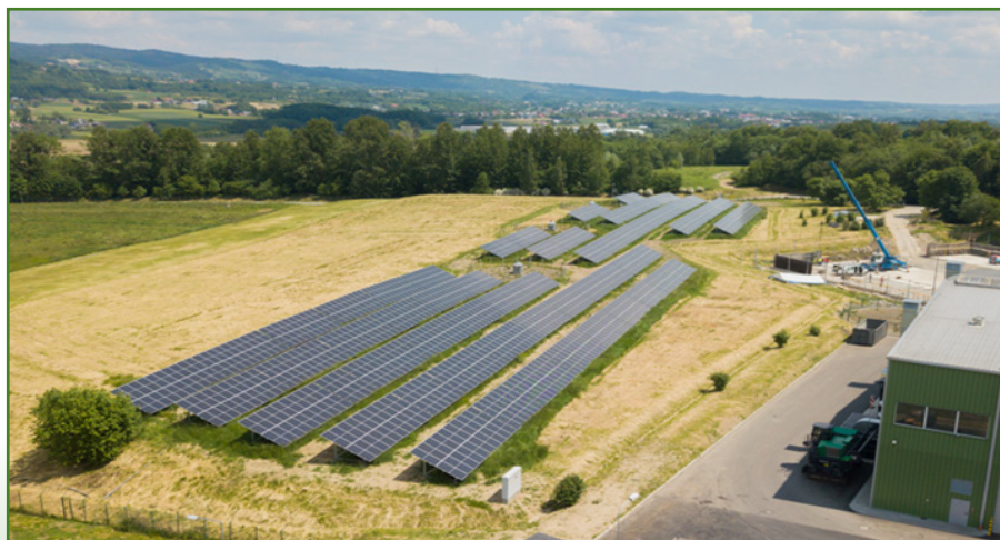
Photo 10. Photovoltaic installation built on the site of the reclaimed landfill in Krosno. Źródło: MPGK Krośnieński Municipal Holding
